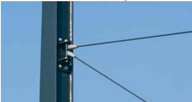
Cable termination on mast
