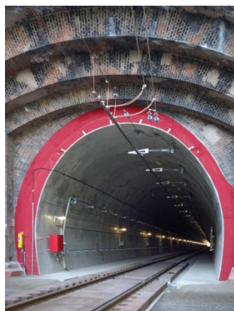
Tunnel with conductor bar. Location: Buschtunnel DE
